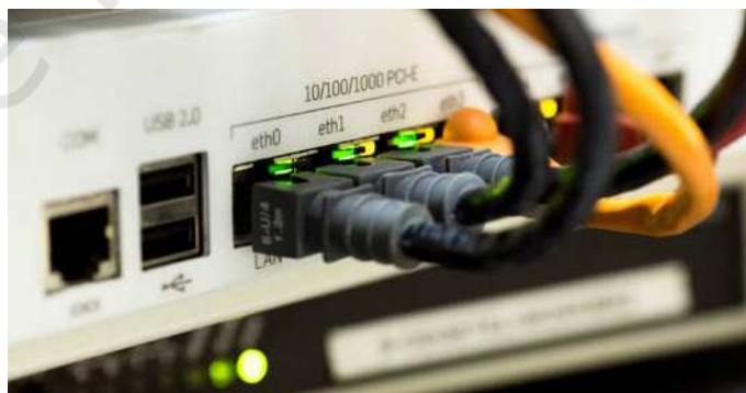
Figure 10.12: Cables connected to a network switch
