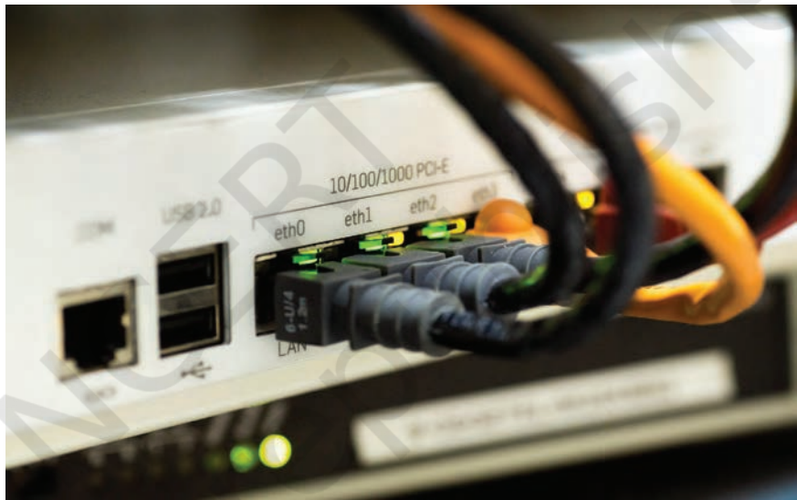
Figure 5.9: Cables connected to a network switch
